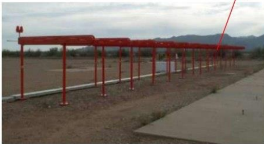
Ground Localizer Antenna
